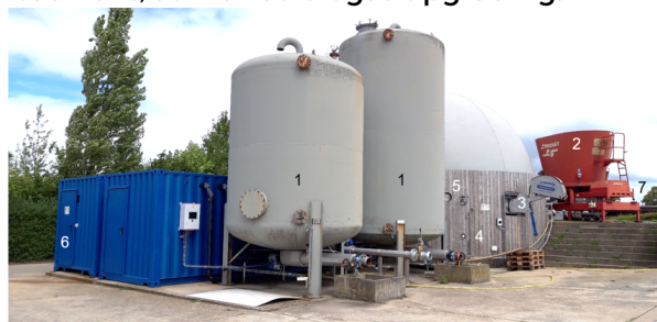
Overview of the biogas pilot plant (Pocket digester (31 kWel)) at Inagro: (1) Silage tanks to store and feed liquid pig slurry; (2) Trioliet screw press to feed the faecal fraction of pig manure; (3) Mixing system; (4) Reactor; (5) Air injection for biological desulphurization; (6) CHP; (7) Partially covered trench silos for the storage of the faecal fraction of pig manure.
