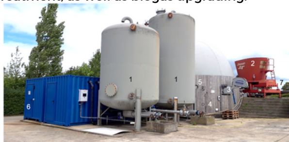
Overview of the biogas pilot plant (Pocket digester (31 kW)) at Inagro: (1) Silage tanks to store and feed liquid pig slurry; (2) Trioliet screw press to feed the faecal fraction of pig manure; (3) Mixing system; (4) Reactor; (5) Air injection for biological desulphurization; (6) CHP; (7) Partially covered trench silos for the storage of the faecal fraction of pig manure.
